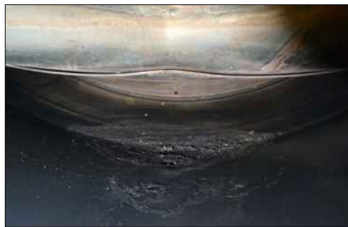
View from inside of the Exhaust Case Drain with Carbon debris
