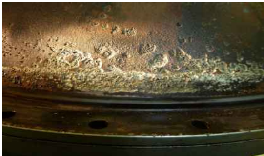
Local corrosion at 6 O'clock
