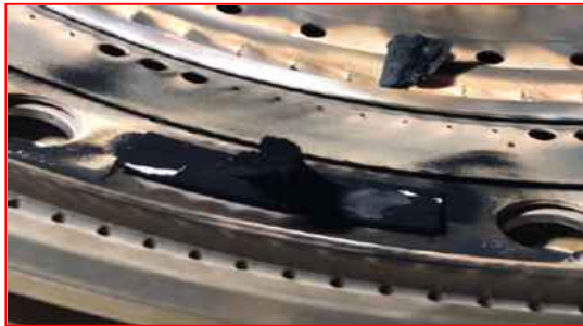
Combustion Chamber – Carbon formation
